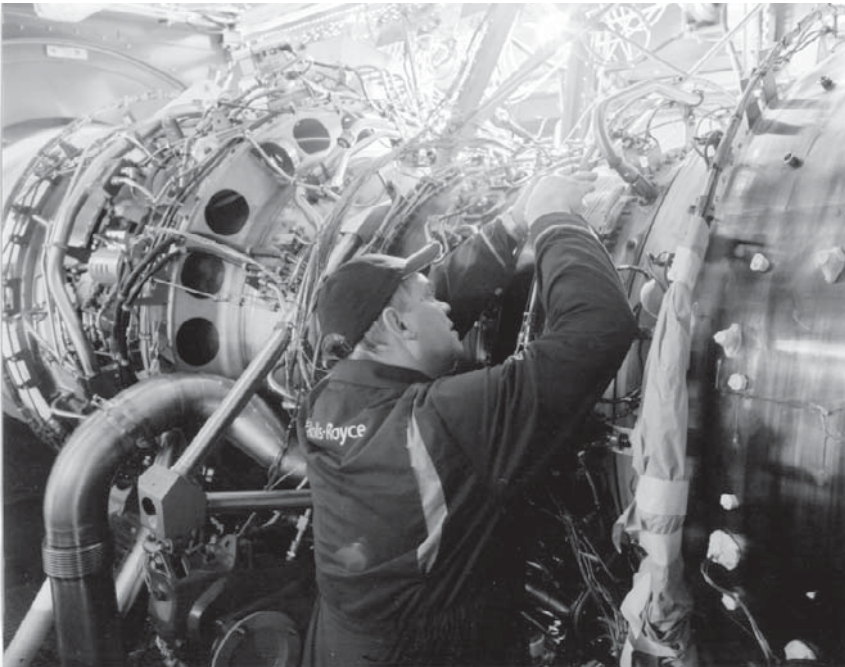
Figure 31.25 Routine maintenance of the Rolls-Royce MT30 gas turbine (shown here on the testbed) is limited to checking fluid levels and visual examinations
